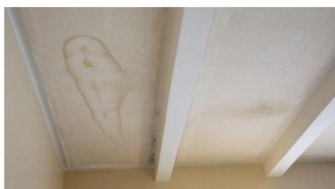
Fuktskada i ljudabsorbent.
